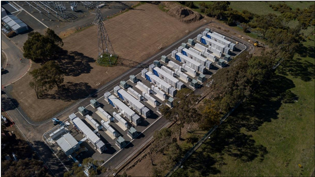
Plate 4-8. Typical battery storage compound configuration ( image reproduced courtesy of Fluence Energy ).
